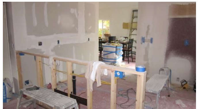
These pictures show our kitchen and family room as work was ongoing. The entire lower level of our home with the exception a single bathroom and the laundry room were gutted and rebuilt.
